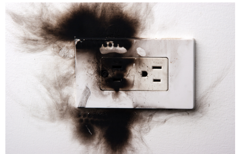
Scorch marks on cover plate
