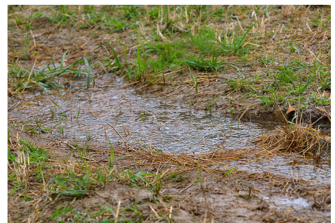
Water pooling in yard; recommend drainage
