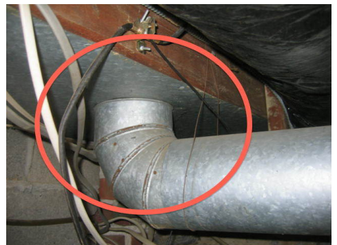
Loose connection; recommend sealing.
